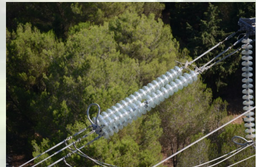
Picture to the right show insulator with broken shed!>>
