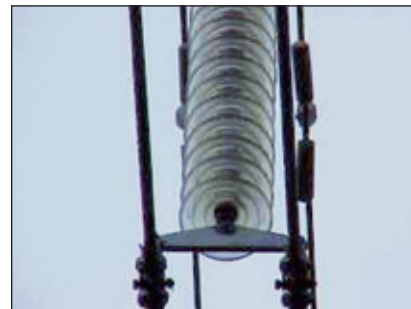
Figure 5 Glass insulator string
