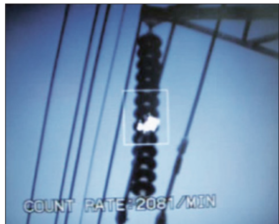
Figure 8 Corona caused by adjacent faulty insulators
